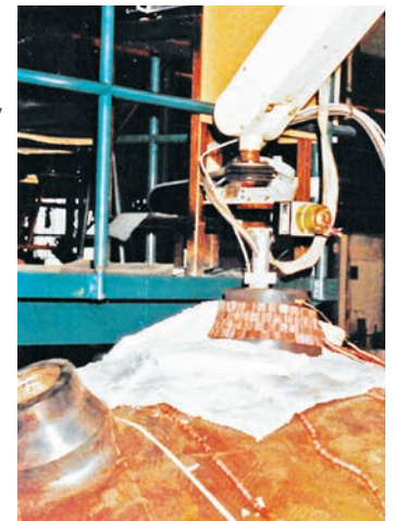
Figure 4: Ceramic electrical resistance elements being used for the internal welding of a pressure vessel head
