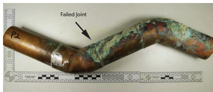
Figure 1: A domestic cold water copper pipe which has suffered leaks from soldered joints. Copyright MCS Ltd
